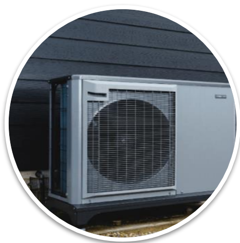
Electric heat pump
